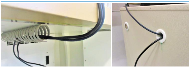
Figure 12: Routing of Power elongation and USB cable.
